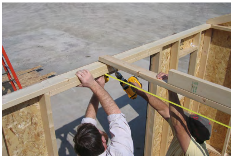
59. Measure the opposite side of the wall before fastening the last temporary brace.
