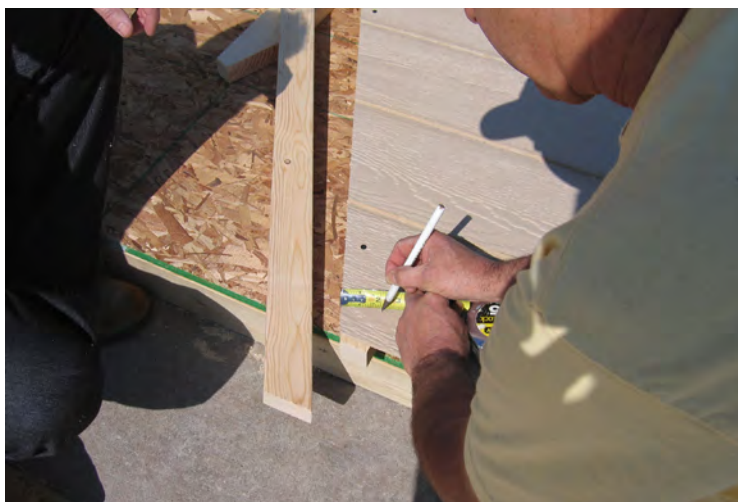
38. For rake installation, measure 2" from the edge of the Smartside siding, and mark with pencil as shown.
