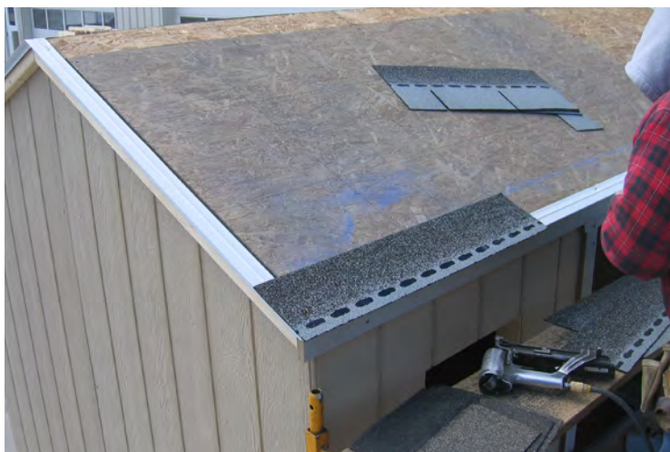
72. Consult the instructions provided with your shingle package. Install the first starter strip along the chalk line as shown.
