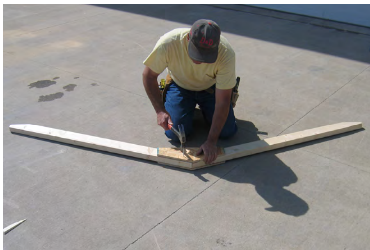
55. Flip the truss around and do the same with the gusset. Repeat with remaining trusses.
