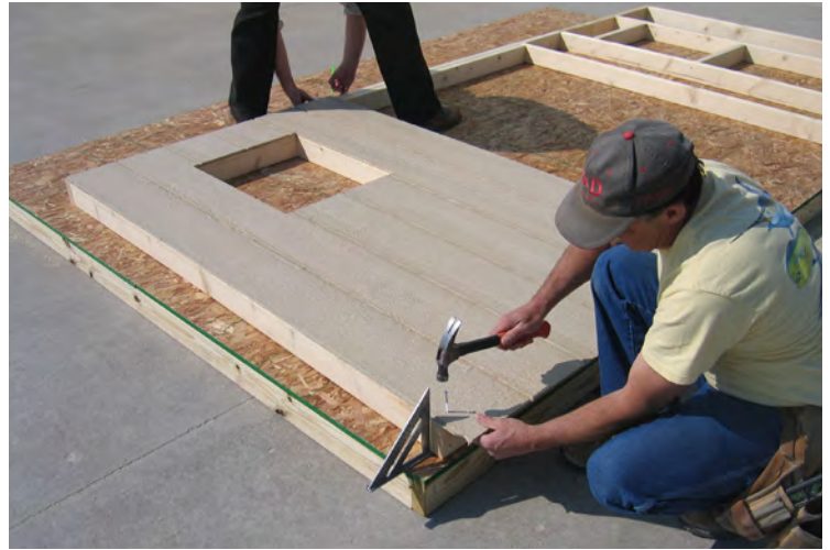
14. Make sure the outside corners are flush as shown before fastening with the 2" nails. Note: There will be a 3" skirt at the bottom.
