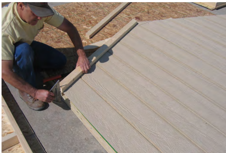
40. Now install the rakes. Keeping them flush at the bottom and secure with 3" nails.
