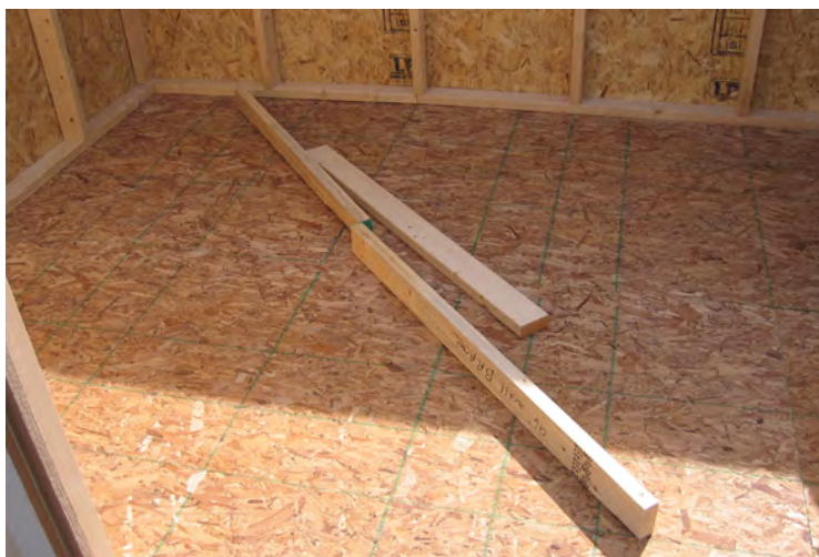
56. Locate the temporary wall braces. Note: Wall bracing pieces may not be included for some smaller buildings, if so, skip steps 56-59.
