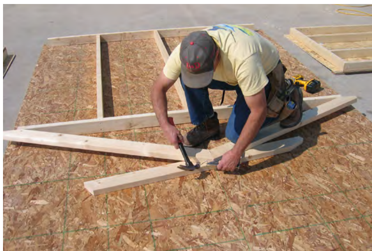
29. Using the WALL LAYOUT DIAGRAM SHEET, locate the truss pieces, layout and fasten with 3" nails as shown.
