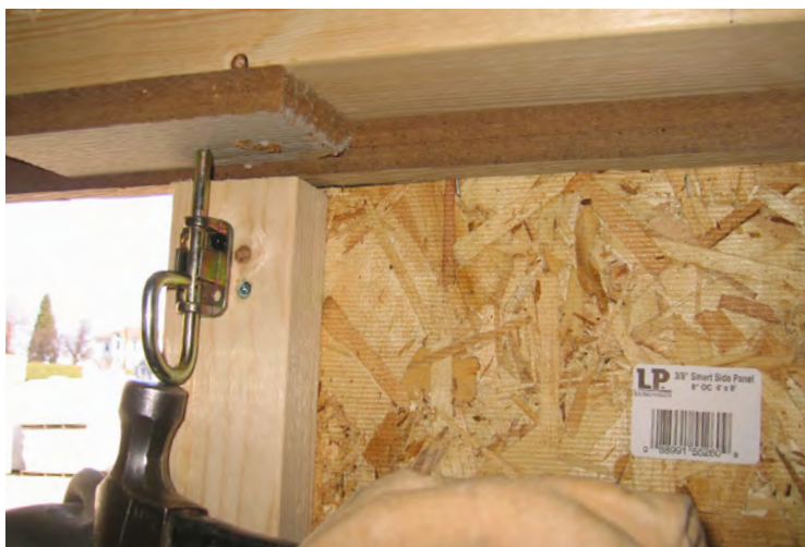
92. Use the hammer again to tap on the top barrel bolt to locate where to drill your 5/16" hole.
