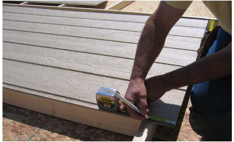
32. Referring to your SMARTSIDE DIAGRAM LAYOUT SHEET. Install the siding on the gable end making sure it is 3" from the bottom of the 2x4 to the bottom of the wall. Note: Gable Sheds will have the doors on one of the gable ends.
