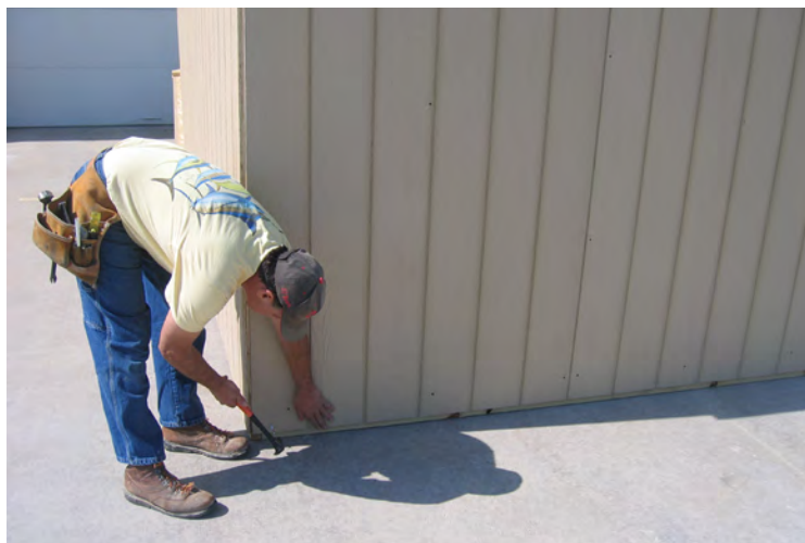
51. Next nail the bottom of the building with 2" nails 8" on center all the way around the building.
