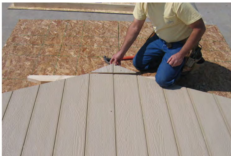
37. Make sure the small piece of Smart side is installed at the top. Repeat with the opposite wall.
