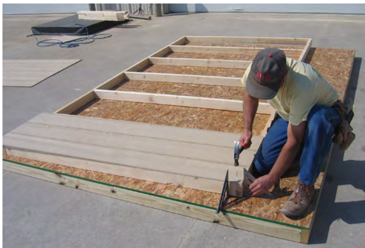
22. Install the Smartside siding, making sure the siding is flush with the 2x4 top plate and end stud.
