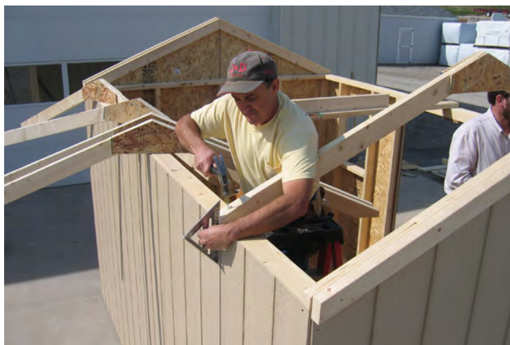
61. Install the trusses as shown, making sure they are 24" on center before fastening with 3" nails. Note: The amount of trusses may vary depending on your building size.
