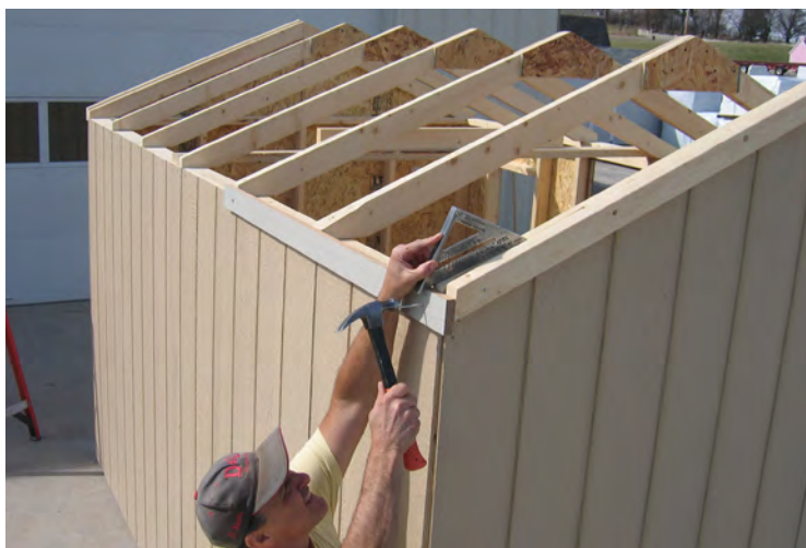
62. Install 2 3/4" trim as shown, keep flush with the outside of the rake and fasten with 2" nails.
