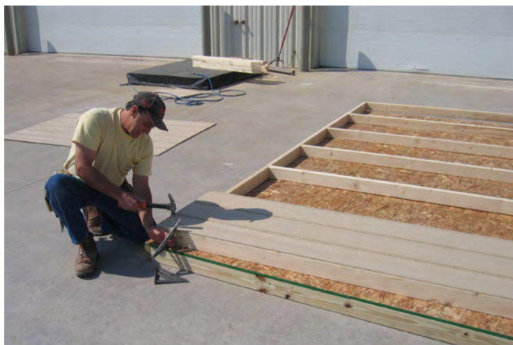
23. Continue installing the Smartside siding. Note: There will be a 3" skirt at the bottom.
