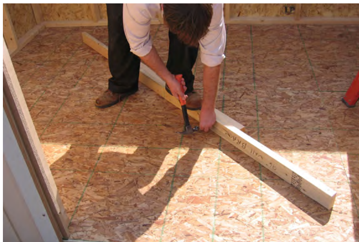
57. Space the temporary wall braces according to the width of the building and fasten them together with 2 1/2" screws.
