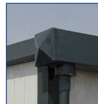
Rear Water Gutter System
